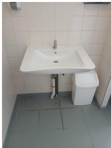
Lavabo accessible PMR
